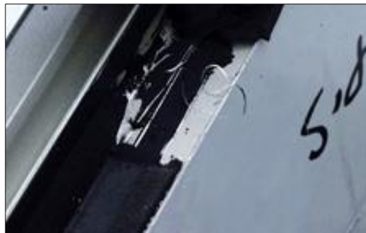
Figure 40: Example with black SG joint - Adhesion failure.
